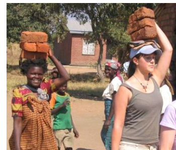
Construction work on a multi-purpose building in Naphini, Malawi was completed in 2007.
